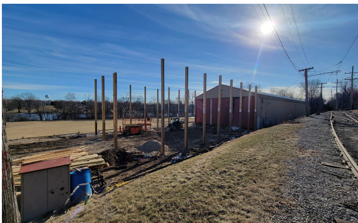
Almost all posts were in for the expanded Fox Valley Trolley Museum barn as of Saturday. A fundraising campaign is underway to bring in the money to complete the project. KATHLEEN JAMIESON
